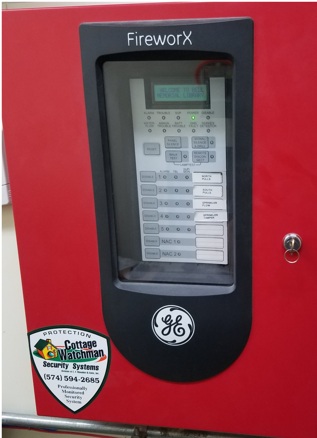
Fire Alarm Panel exterior.
