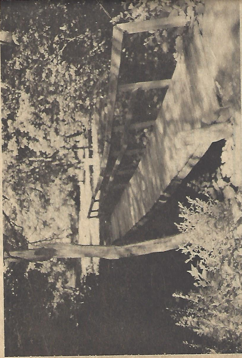
The dangerous old footbridge in Mentzer Park, Mentone, will soon be replaced according to town officials.
